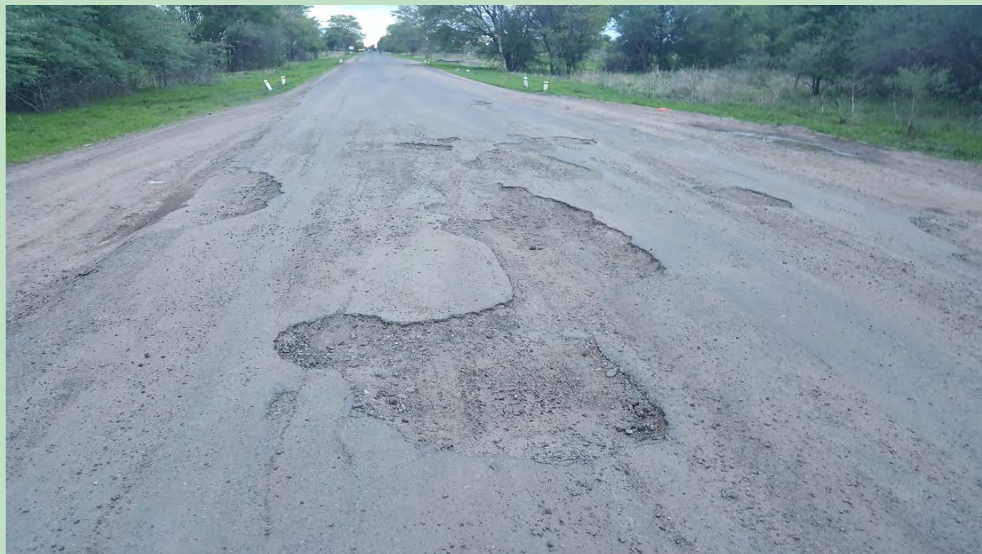
A Road needing repair: This is part of the Kazungula - Sesheke road stretch
