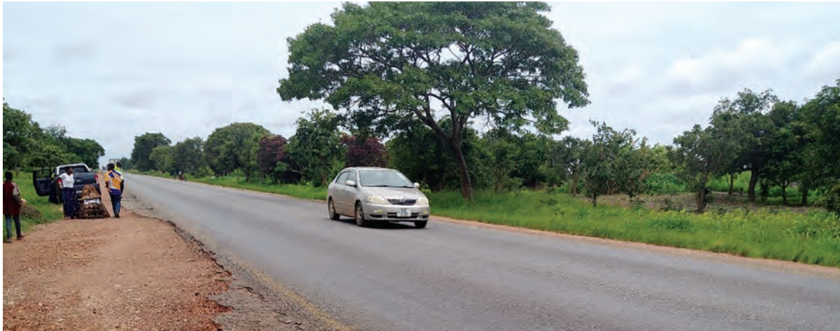
Figure 2: Road Safety Inspections: Road with broken Shoulders
